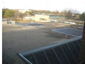
Priority 3 Example Correct ponding issues on roof
