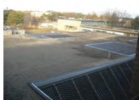
Priority 3 Example Correct ponding issues on roof
