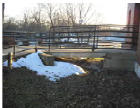
Priority 1 Example Replace deteriorated handicap ramp
