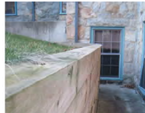
Priority 2 Example Repair retaining wall
