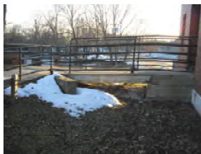
Priority 1 Example Replace deteriorated handicap ramp
