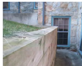
Priority 2 Example Repair retaining wall
